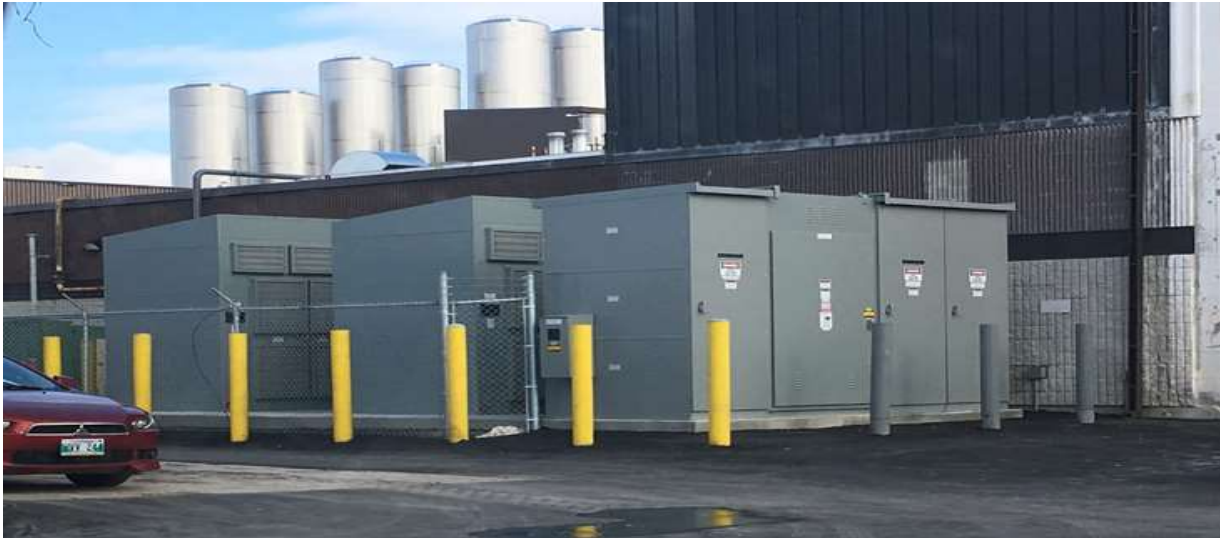
Figure 1: Outdoor dry type Transformer 3750 kVA, Winnipeg, 2017.
