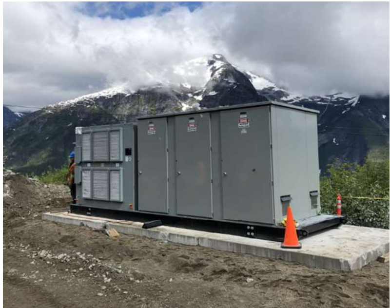
Figure 4: Dry type transformer, 10000kVA, British Columbia 2015.
