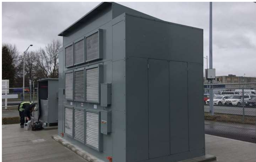
Figure 3: Outdoor Sept Up Transformer ( 4,160 to 24,440 V), Vancouver airport 2018.
