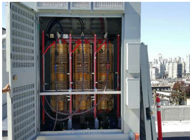
Figure 2: Dry type Transformer 2 000 kVA, Vancouver 2016.
